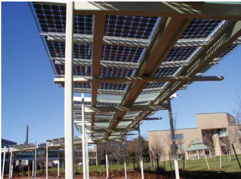
PV panels shade the MITRE Corporation' of Bedford's walkway while generating 15.4 kW of electricity. 9.6 additional kW are installed on the building's roof.
