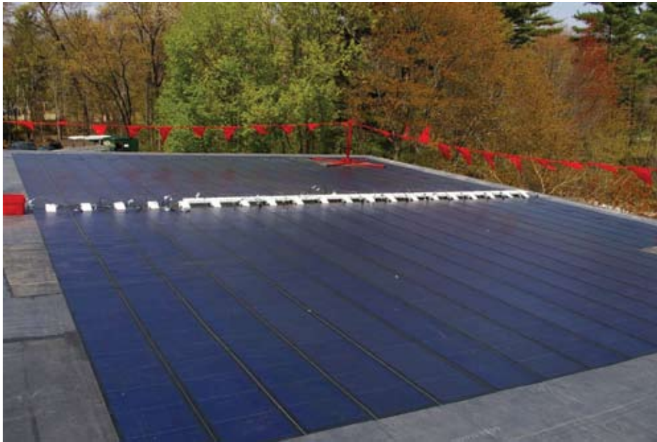
16-kW thin film solar electric laminate array at MI Realty of Leominster
