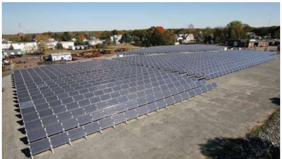
460-kilowatt Brockton Brighfield project on former brownfield site
